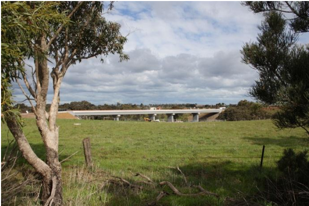
Figure 6. RRL construction over Werribee River along the western boundary of the Riverdale PSP.
