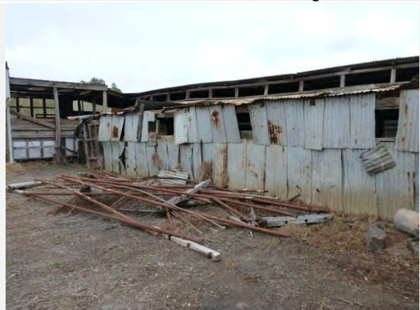
Property 44 Dilapidated sheds containing suspected ACM.
